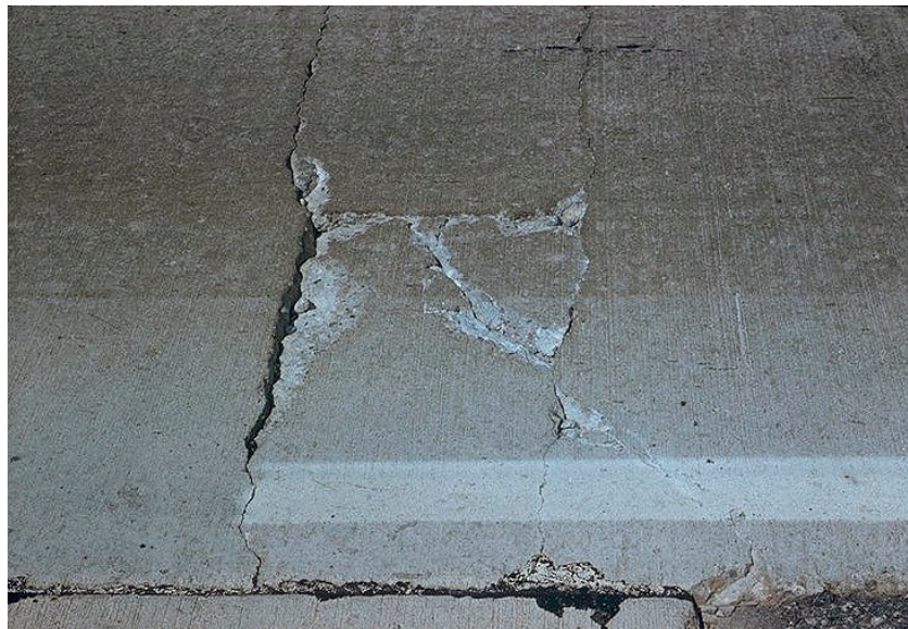
Figure 64. Typical CRCP punchout distress.
