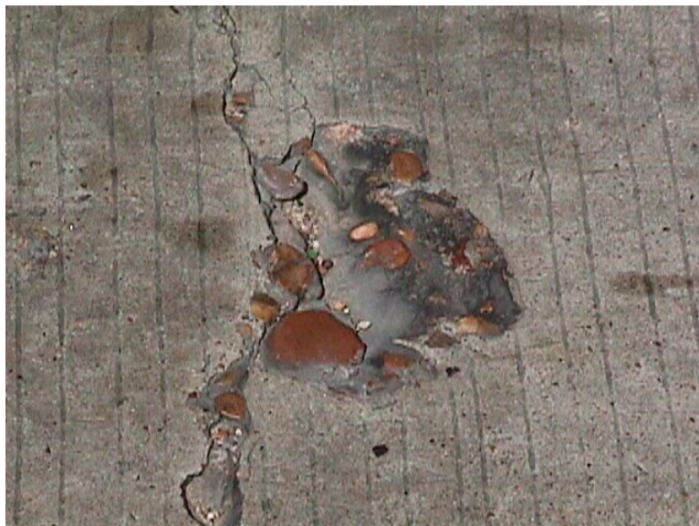
Figure 54. Round-shaped aggregates at a spalled CRCP crack.
