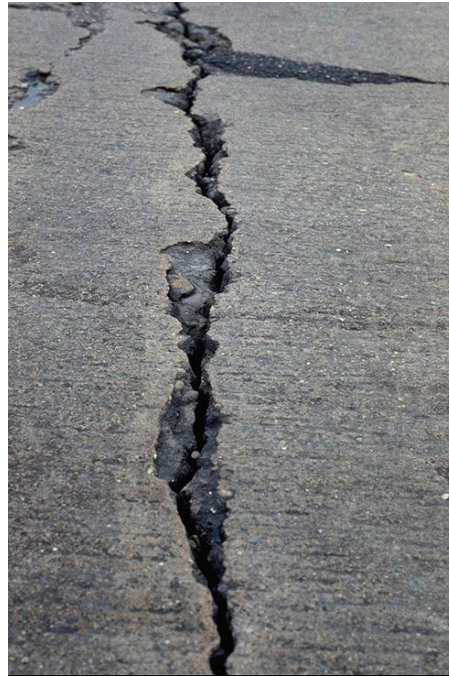
Figure 59. Photograph of deflection spalling on a CRCP.
