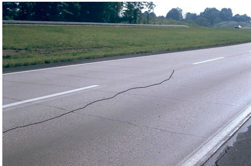
Figure 20. Longitudinal crack in CRCP due to thermal shock. Crack is enhanced for clarity.
