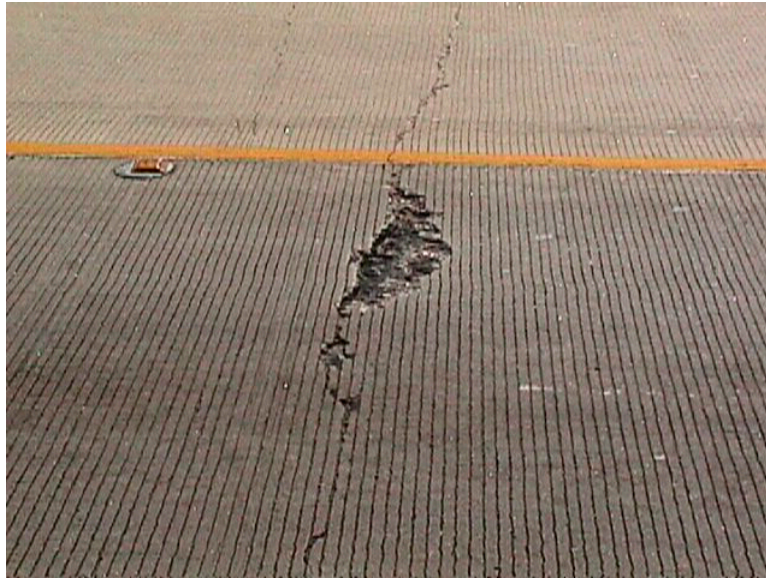
Figure 53. Delamination spalling at a CRCP crack.
