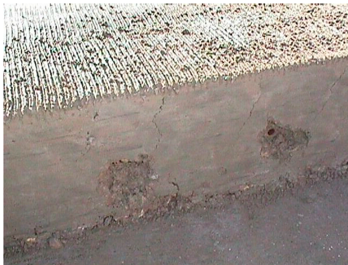
Figure 18. Plastic shrinkage cracking in concrete pavement.
