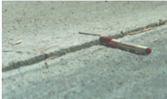
Figure 26. Photograph of faulting in JPCP.
