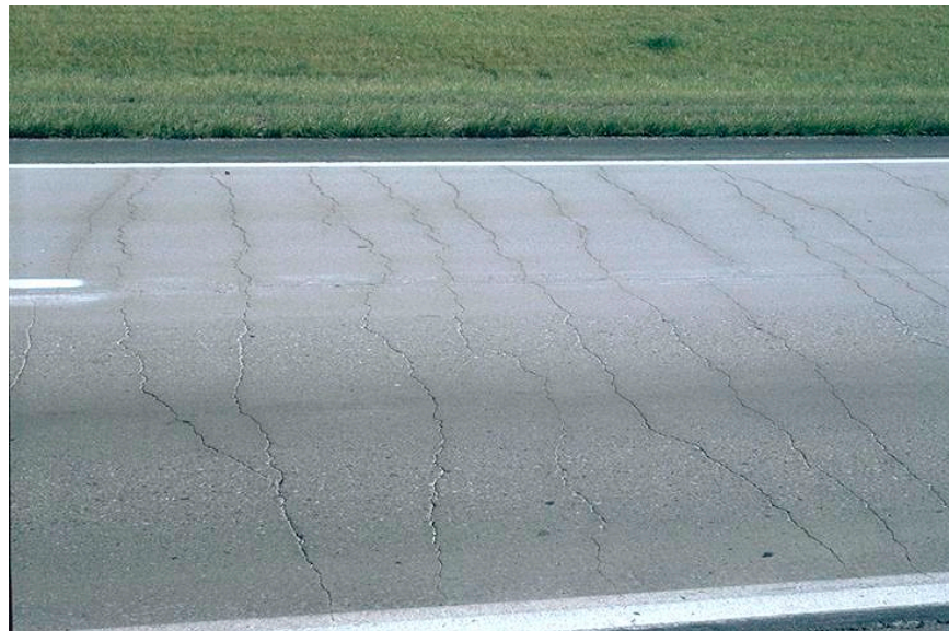
Figure 19. Closely spaced cracks resulting from thermal shock in CRCP.
